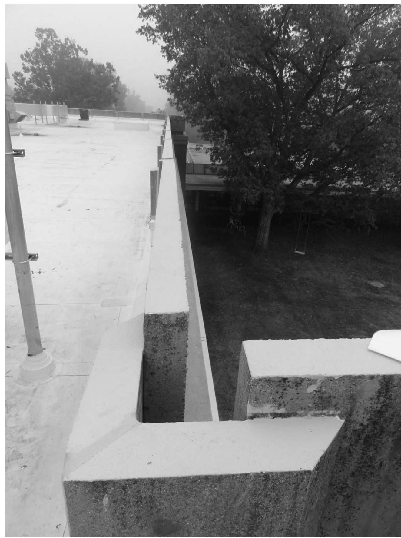
STANLEY HALL PARAPET EXISTING CONDITIONS PHOTO TYPICAL TOLERANCE / ALIGNMENT OF EXISTING PANELS
